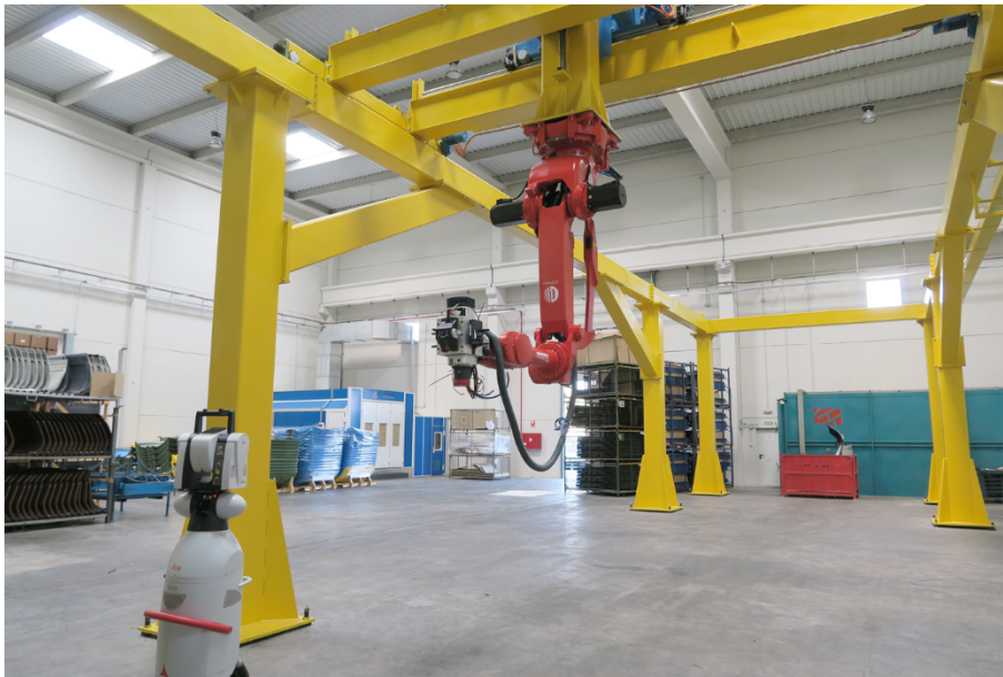
Fig. 1. Prototype system with CSEM control and Leica tracking system (installation at AITIIP, Zaragoza, Spain).
