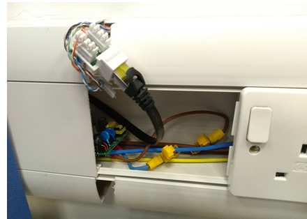
(b) The prototype attack device in situ inside service trunking on an office wall.
