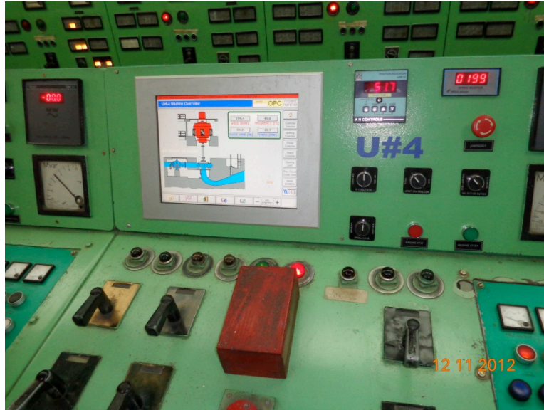
Fig. 2. Control Room Panel of a Hydropower Plant
