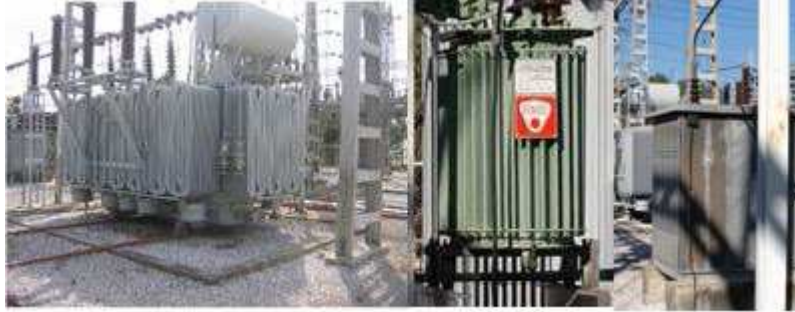
Fig. 2. Protected substation components: HV/MV Power Transformer (left), Neutral Reactance (centre) and Neutral Resistor (right).
