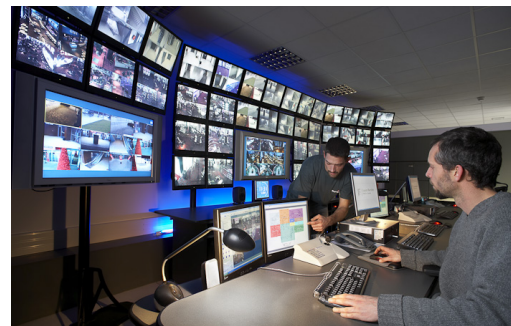
Figure 2. A control room for video surveillance (source [30])
