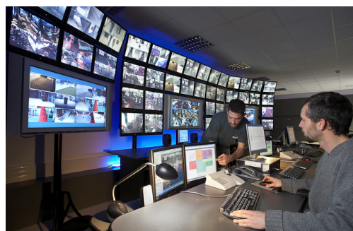
Figure 2. A control room for video surveillance (source [30])
