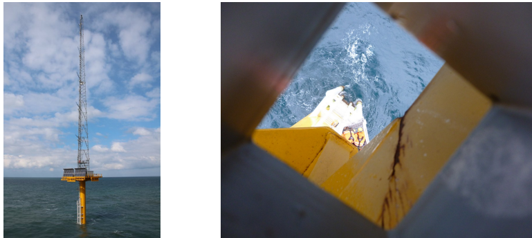
Figure 1: Offshore meteorological mast (left). Cracks in a offshore platform (right). Both pictures available by the courtesy of Universal Foundation A/S.
