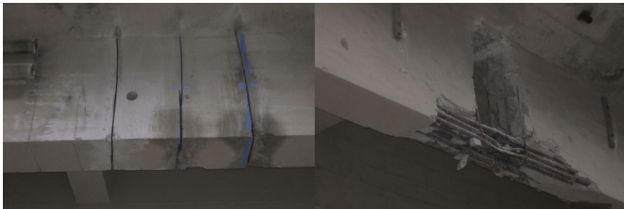
Figure 7.14: Artificial damage induced to side beams (damage 1) and centerline of the bridge (damage 2).
