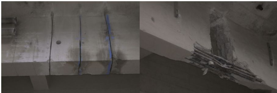
Figure 7.14: Artificial damage induced to side beams (damage 1) and centerline of the bridge (damage 2).
