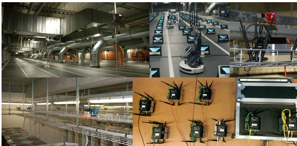
Figure B.6: Hardware employed in the testbed and the scenario where it is deployed.
