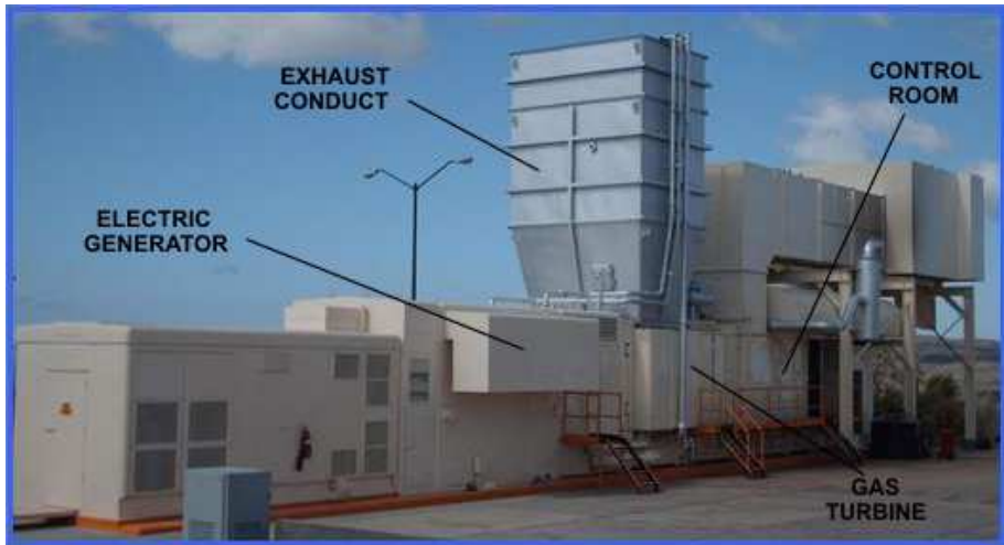
Figure B.2: Turbo-Generator at the Chankanaab Turbo-Gas Central.
