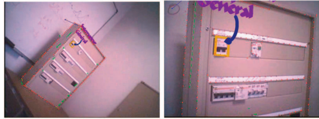
Fig. 6. Tracking of an electrical panel: illustration of the dynamic modification of the model (some parts are added or removed according to the relative camera/object position).
