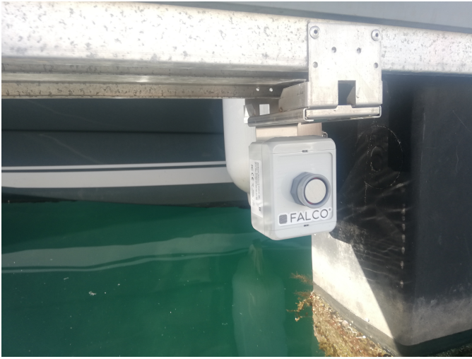
Fig. 2. Falco Presence sensor riveted on the pontoon to monitor presence of a boat at the specific slip. The sensor is located below the pontoon floor level.
