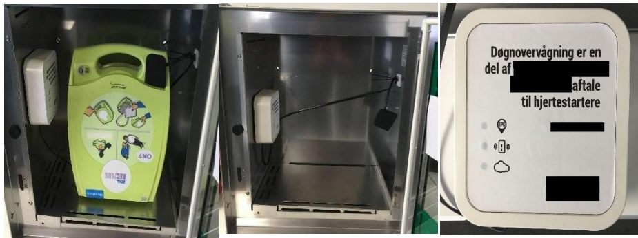
Fig. 4. Left: AED inside the cabinet. Middle: The monitoring unit and “optical eye.” Right: The monitoring unit.
