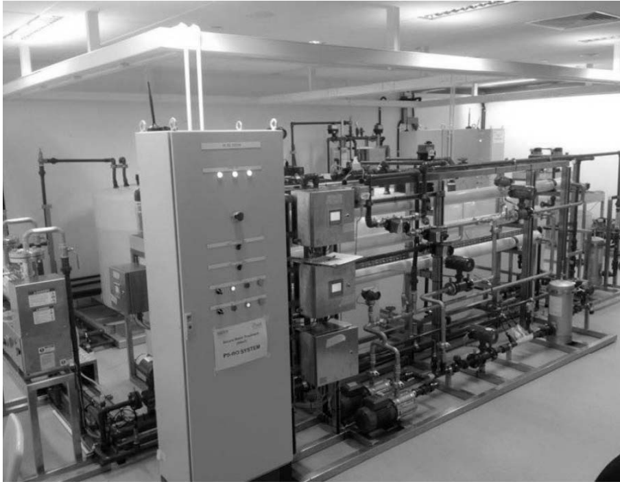
Figure 1. Secure Water Treatment (SWaT) testbed [3].
