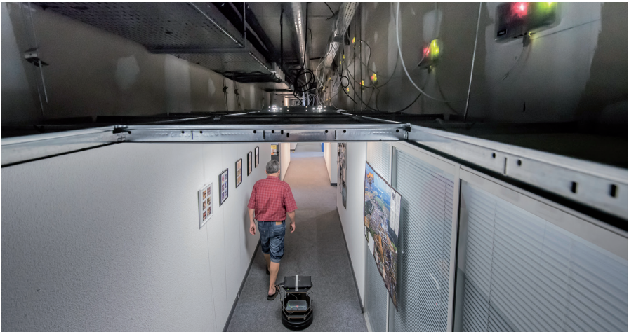
FIT/IoT Lab sensor network installed in the Inria Grenoble Rhône-Alpes research center. © Inria / Photo H. Raguet.
