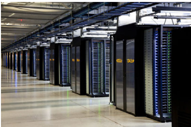
FIGURE 7.9 — Data center FACEBOOK.
