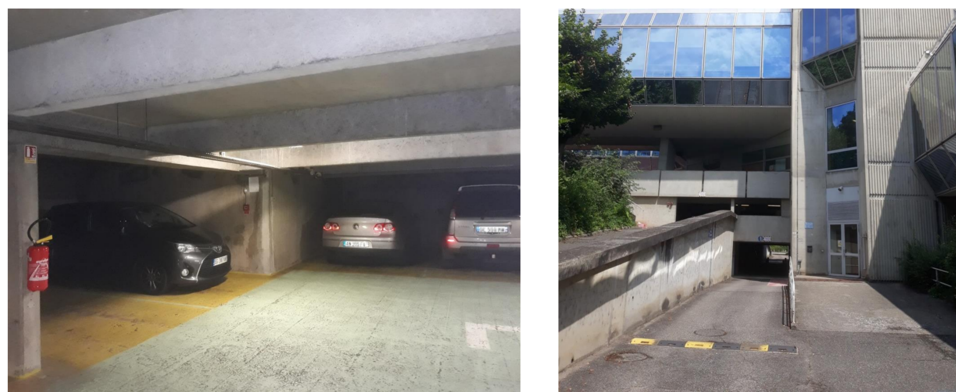
Example of concrete structure environments of underground parking sensors parking in Orange Labs Meylan
