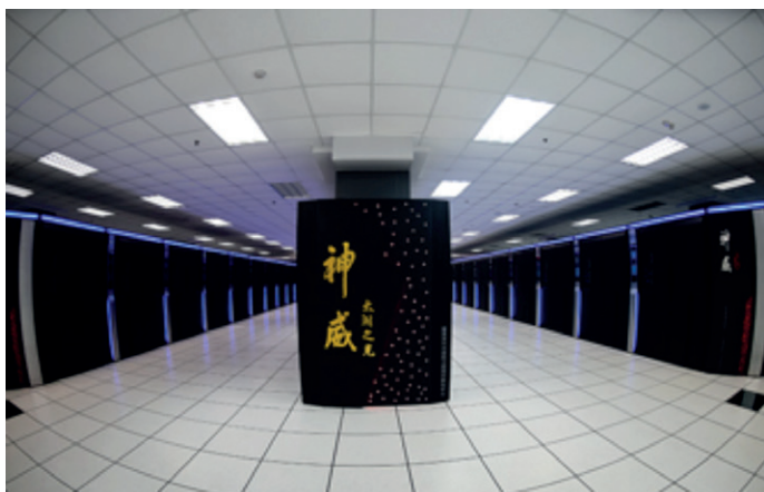
Figure 147: Sunway TaihuLight Source: Xinhua
