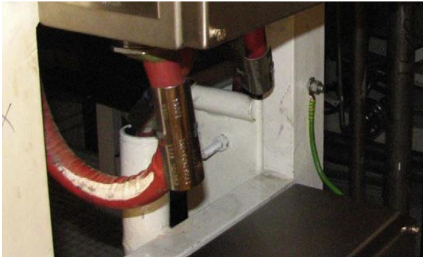
Fig. 2. High mechanical bending stress on NPP power cable [4].
