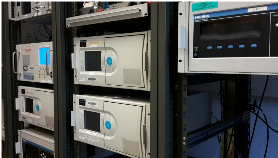
Figure 2 A set of analyzers as they are typically found in a fixed station
