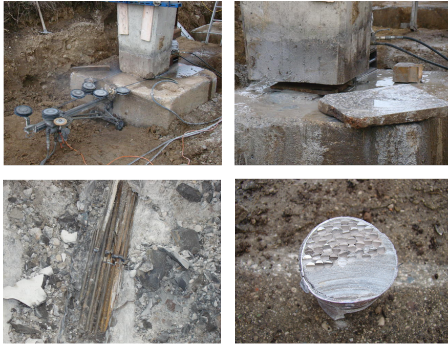
Fig. 7 Progressive damage of column and tendons on bridge S101 [23].
