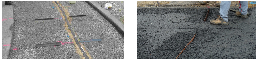
Fig. 2 Photographs showing the different types of steel bars embedded in the asphalt.
