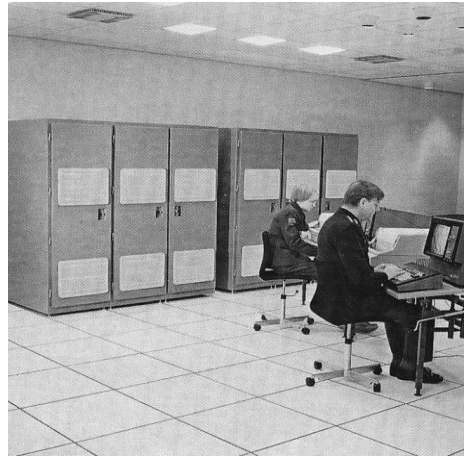
Fig. 7. Typical CAMPS Installation
