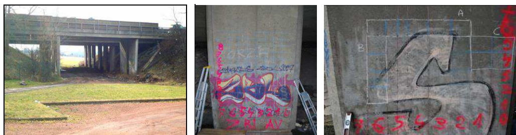
Figure 5 : On site test and example of identification of the measurement zones a) Structure b) Prior auscultation pattern c) Auscultation zones
