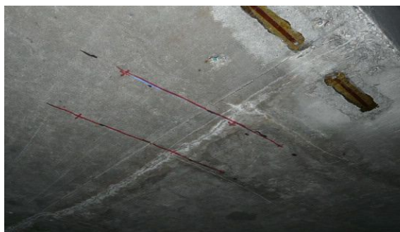
Figure 3: Transverse crack and marking of tendons in the lower slab
