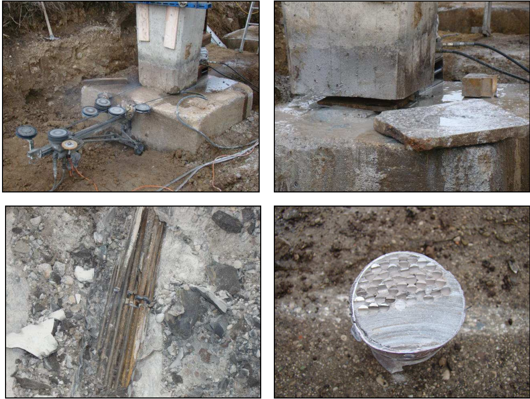
Figure 2. Progressive damage of column and tendons on bridge S101 [25].
