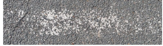
Fig. 10: Old road marking with time wear
